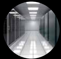
Precision Air Conditioning
